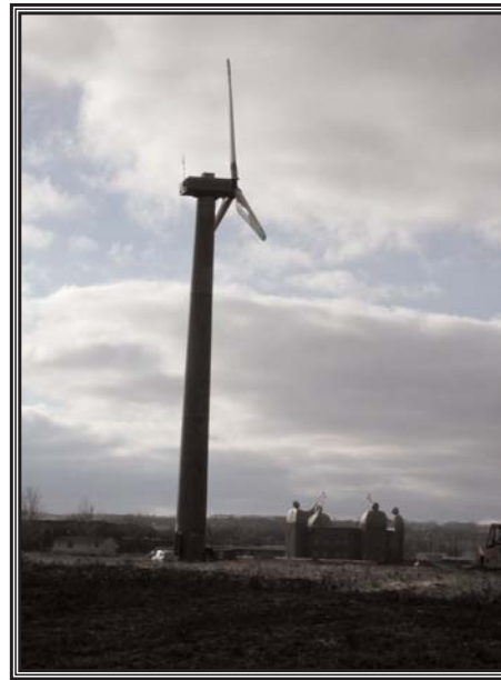
(New) Wind Turbines at SWC
